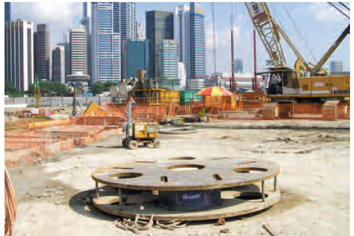
A single level three O-Cell setup ready to assemble in a reinforcing cage.
